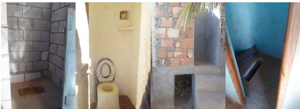
Figure 5: New dry toilets in Beni Isguen (2019)
